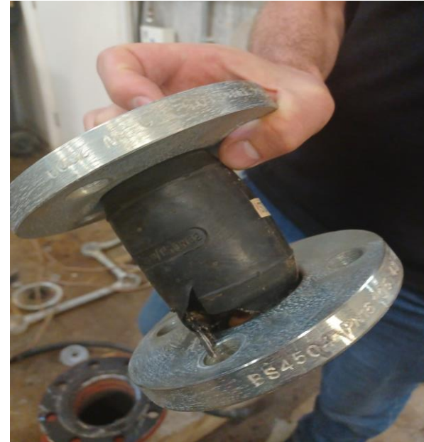
Burst bellows causing heat network outages
